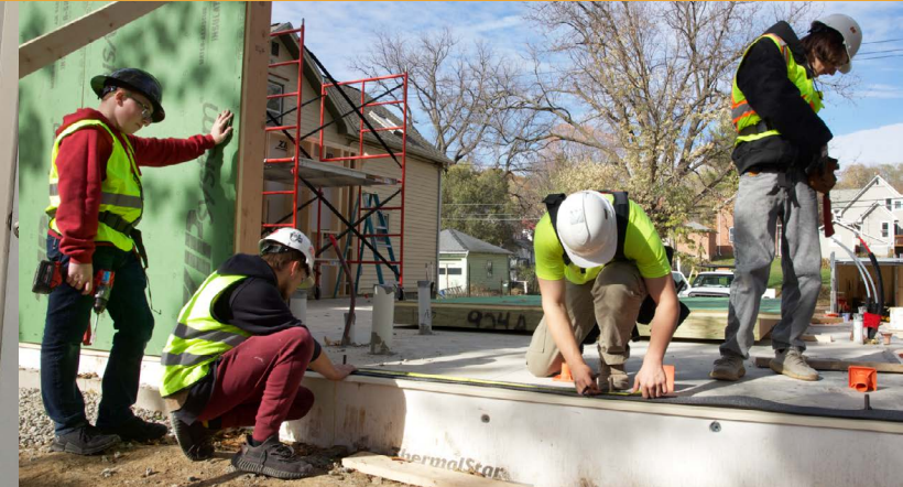
Ronalds St. – Student built house in partnership with the ICCSD, HBA Vocational Training Council, and The Housing Fellowship
