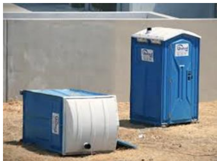
Position portable toilets so that they are secure and will not be tipped or knocked over. Photo credit: Kentucky Best Management Practices for Construction Activities, 2005
