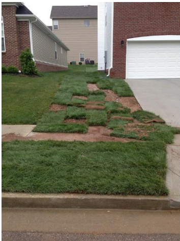
Sod installation failure. Sod needed staples. Photo credit: Barry Tanning, Tetra Tech
