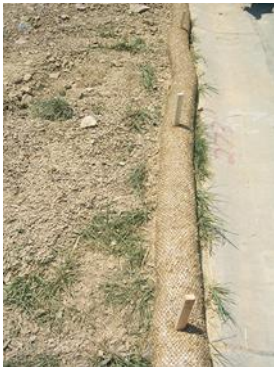
Drive stakes every 3-4 feet along the filter log. Photo credit: Barry Tanning, Tetra Tech.
