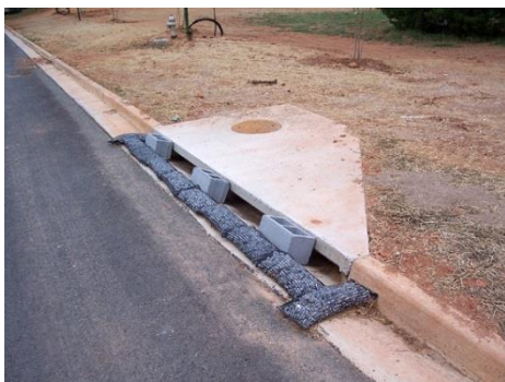
Typical rock bag inlet protection installation. Photo credit: Barry Tinning, Tetra Tech
