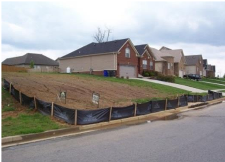
Site with properly installed silt fence. Note that fence posts are installed on the downhill side of the fabric. Photo credit: Barry Toning, Tetra Tech
