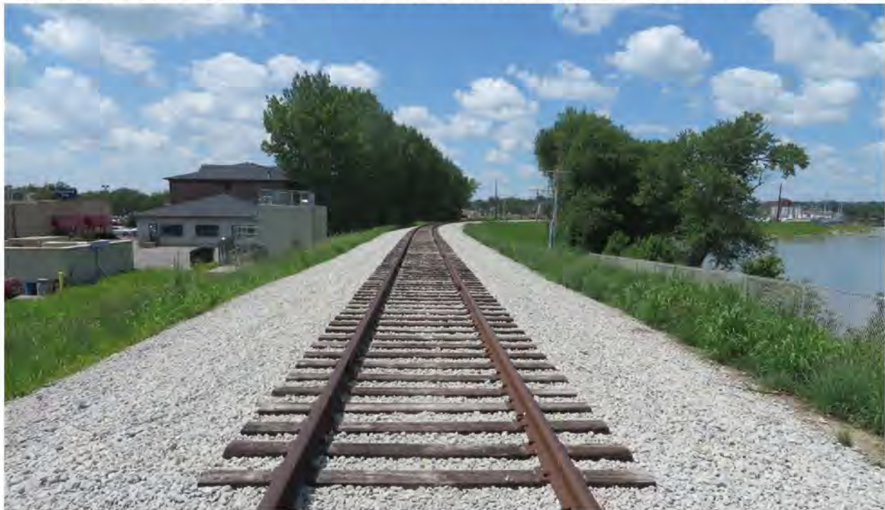
Figure 8: CRANDIC Corridor Main Track Structure near Rocky Shore Drive in Iowa City
